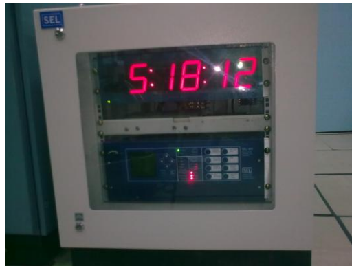
Fig 4 - PMU and GPS at Sub-station
