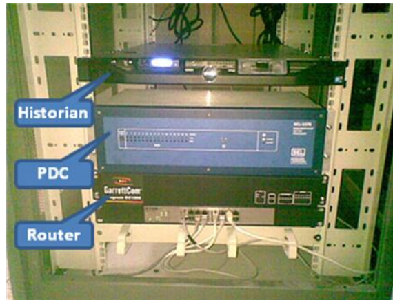
Fig 3 - PDC and other equipments at NRLDC
