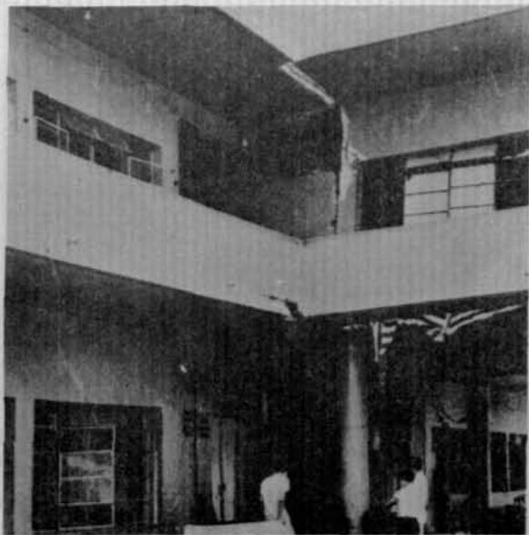
DAMAGED SCHOOL FIGURE 16
