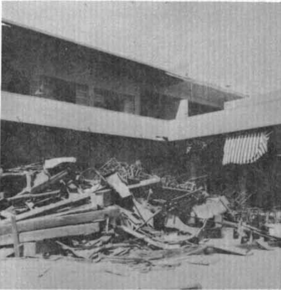
PARTIALLY COLLAPSED SCHOOL FIGURE 15
