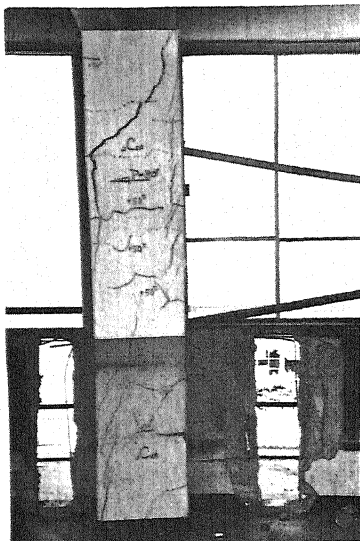
Photo 7. Shear Cracks in 2nd Storey Interior Column (Maibara).
