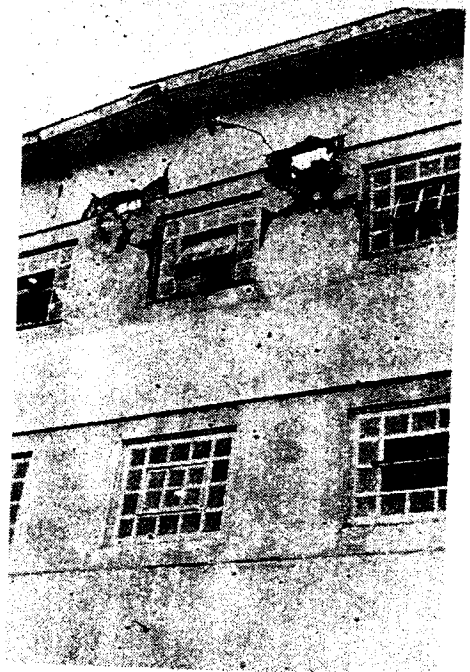
Fig. 1.94 Ditto. Detail of failure in parapet.
