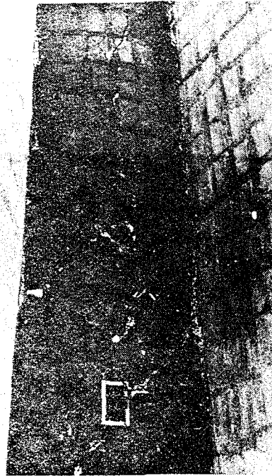
Fig. 1.46 Ditto. Damage in cylindrical ventel wall.
