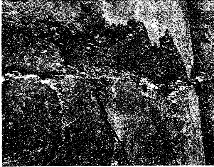
Fig. 12.- Volcan Silo. Detail of horizontal crack.
