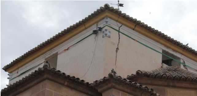
Figure 8. Damage and emergency confinement on the walls that surround the dome of I3.
