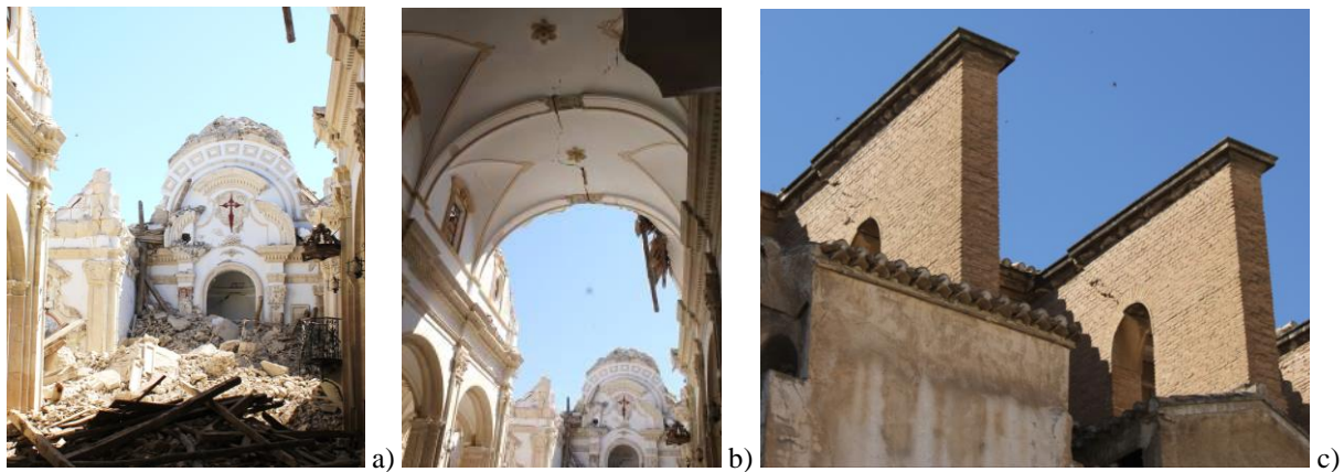
Figure 4. Damages to I2 after the collapse of the chancel and of the transept area, including the dome (a) and (b), and extensive cracking of the buttresses (c).
