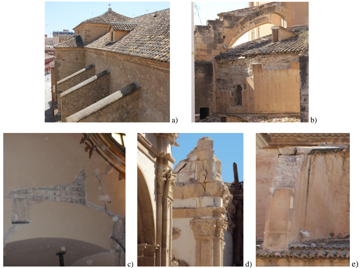
Figure 3. Masonry type M1 at the church of San Francisco (a), M2 at the cathedral of San Patricio (b), M3 at the chapel of N. a Sr. a do Rosário (c), M4 at the church of Santiago (d) and M5 at the cathedral of San Patricio (e).
