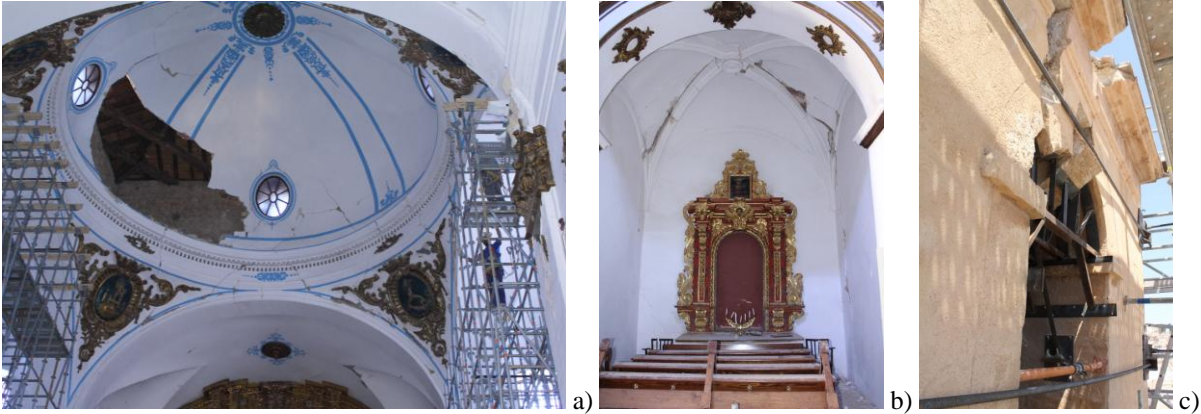
Figure 7. Damages to the dome (a) and lateral chapels (b) of I5, and vertical displacements of the keystone of one of the belfry arches of the tower (c).
