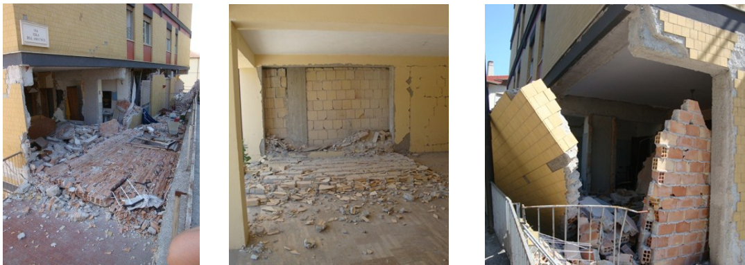
Figure 2. Failure patterns of masonry infill walls found in the recent earthquake of L'Áquila
