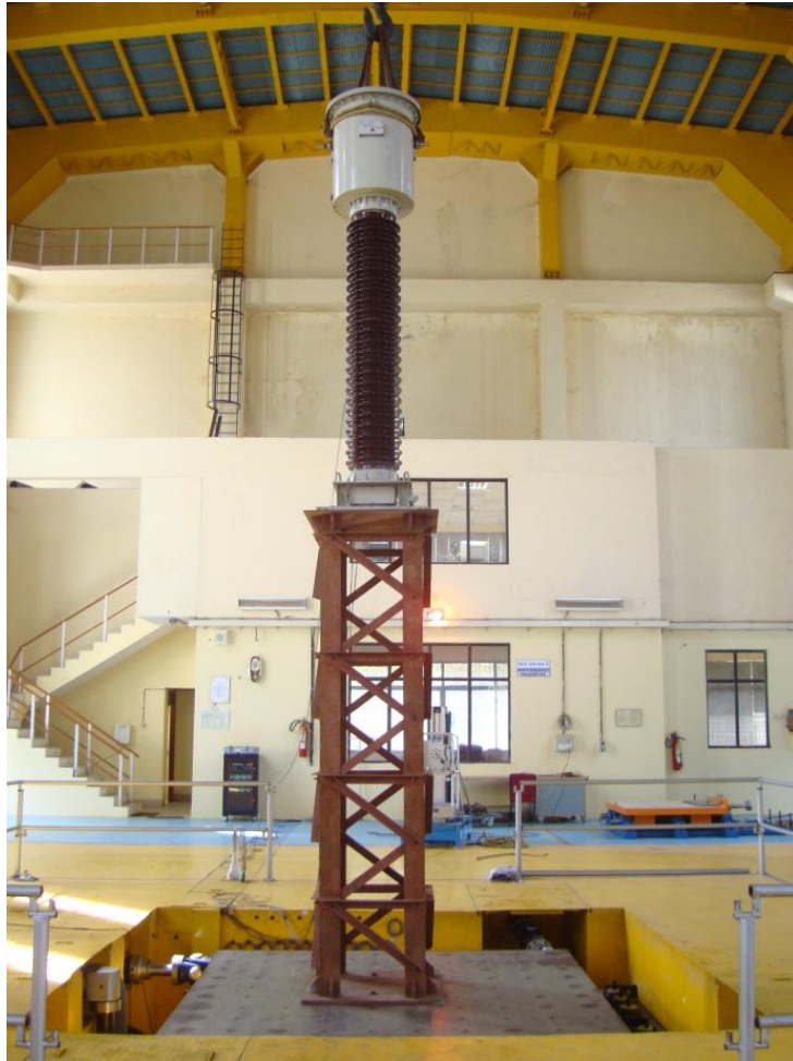
Figure 3.1. Instrument Transformer mounted on Shake Table.
