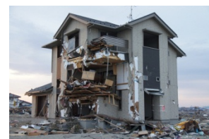
Photo 2.14. Remained 3-story wood house.
