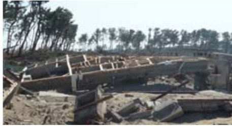
Photo 2.1. Foundations washed away.
