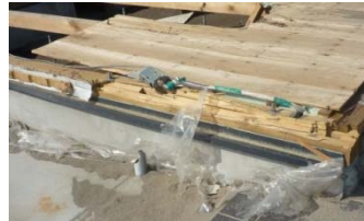
Photo 2.4. Sills, foundations and floor boards remained.
