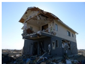
Photo 2.11. Remained house which didn't have survived buildings in the inundation direction.
