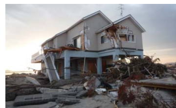
Photo 2.12. The remained hybrid construction consisting of RC for the 1st floor and wood construction on the 2nd floor.
