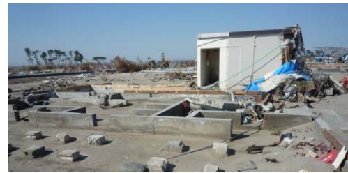
Photo 2.2. Only foundation remained.
