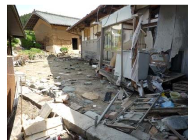
Photo 2.19. Survived old house which rotated and moved horizontally
