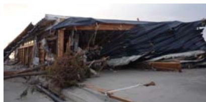
Photo 2.13. Remained glulam frame structure.
