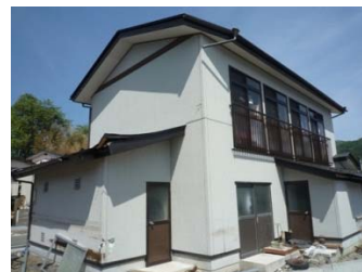
Photo 2.16. Wood house without damage under the flood water depth of over 7 m.
