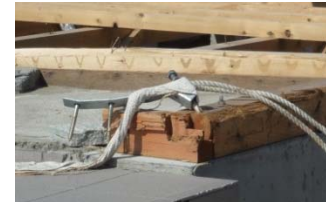
Photo 2.5. Failed hold down fastener.
