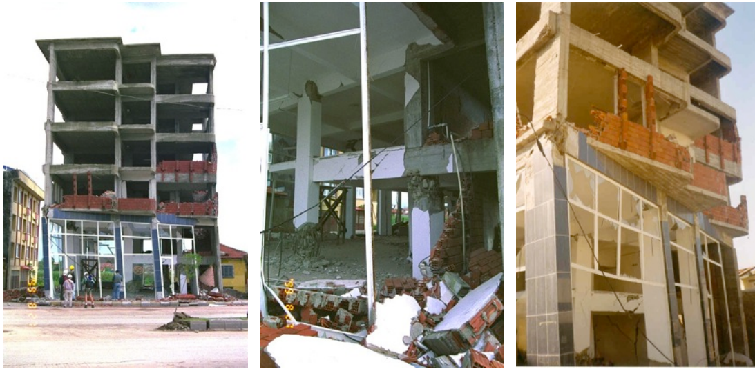
Figure 10. Overview of the damages of the 2 nd case study structure
