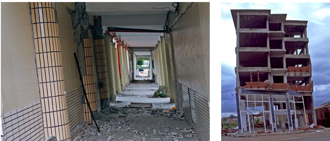
Figure 1. Examples of buildings with large residual displacements that typically lead to demolition (left photo by M. Bruneau, MCEER; right photo by A. Whittaker, NISEE, EERC, UC Berkeley).
