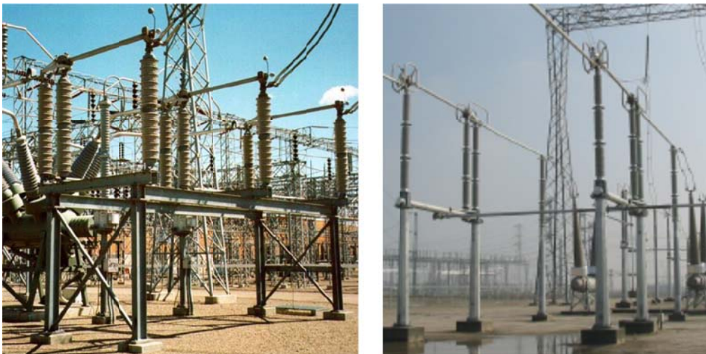
Figure 1.1 Typical field installation of 230-kV (left) and 550-kV (right) electrical disconnect switches.
