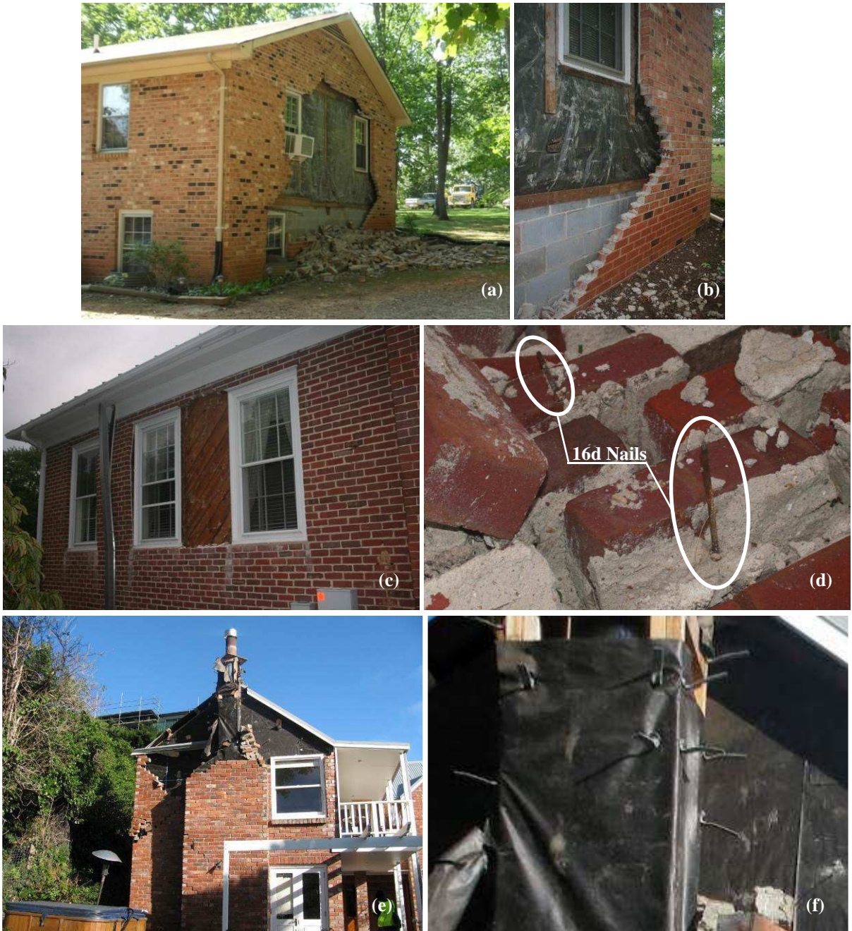
Figure 1. Brick veneer wall damage and collapse following earthquakes in (a-d) August 2011, Mineral, Virginia (photos by Matthew Eatherton, Virginia Tech), and (e,f) February 2011, Christchurch, New Zealand (photos by Kevin Jackson, Thornton Tomasetti).
