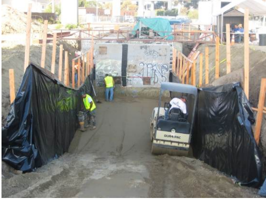
Figure 3.2. Compaction of backfill material with vibratory roller and hand whacker in T 2.4,1
