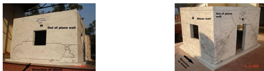
Figure 5.3. Damage to bending (cross) walls of Model 1 on west and east side after shock 4
