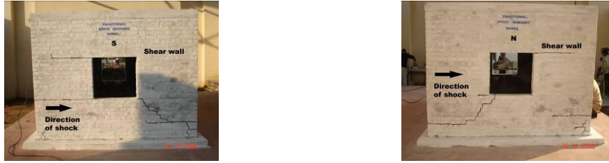
Figure 5.4. Damage to shear walls of Model 1 on south and north side after shock 4
