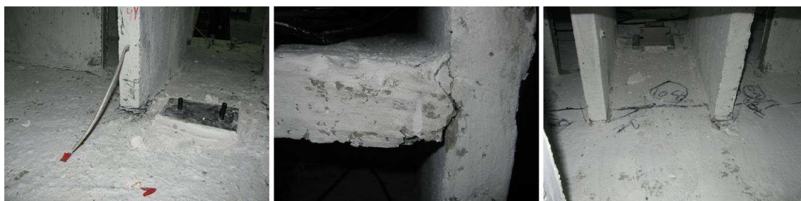
Figure 4.1. Damages at the walls above the foundation, wall – slab connections and first story slab.
