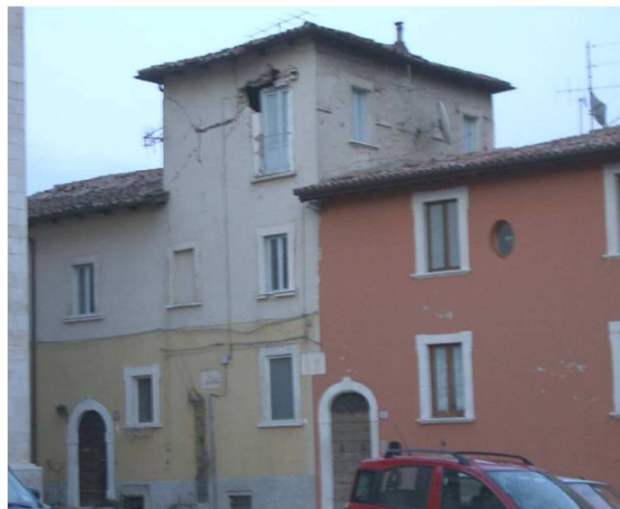
Figure 6. In plane damage of third story due to different heights of adjacent buildings after the 1999 earthquake in L'Aquila (source: Calderoni et al, 2009).
