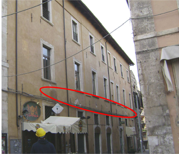
Figure 2. Diagonal cracks (shear failures, surrounded by the red line) on the spandrels of a masonry building in l'Aquila. The global failure mechanisms of the façade have been prevented through the iron ties, and only local failures are observed (source: Calderoni et al, 2009).
