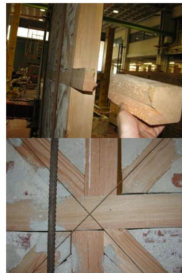
b) Failure by parallel shear of intermediate timber beam for MW2
