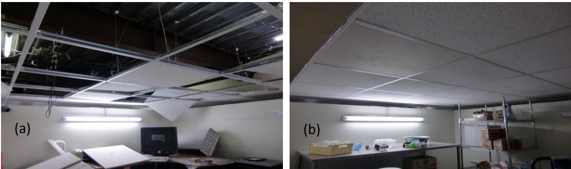
Figure 9. Condition of (a) braced ceiling (5 th floor) and (b) unbraced ceiling (4 th floor) after 3D-Northridge-Rinaldi (TPB system)
