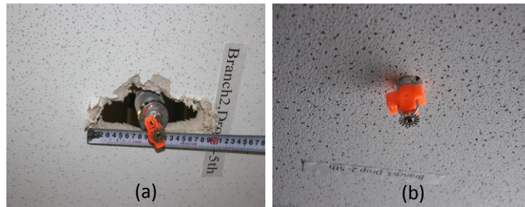
Figure 17. Comparison of observed damage near (a) conventional sprinkler head, and (b) flexible hose sprinkler head after 2D-Tohoku-Iwanuma (base fixed)
