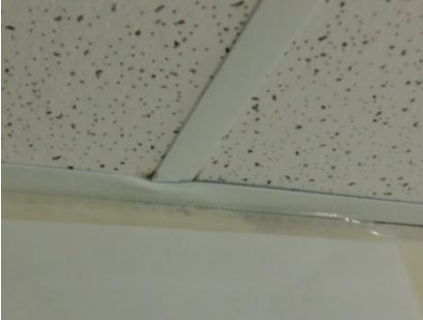
Figure 13. Ceiling perimeter attachment failure after 3D-Northridge-Rinaldi (TPB system)
