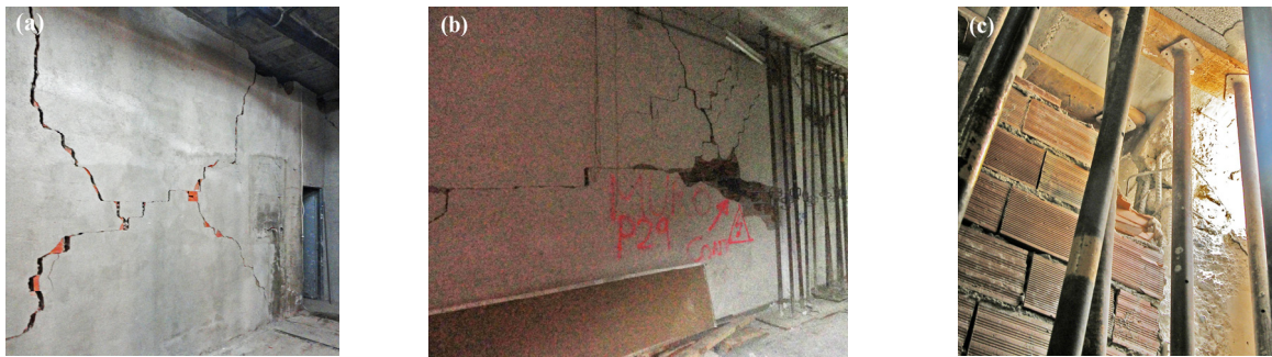
Figure 7. In-plane failures in masonry infill panels: shear diagonal cracking (a), horizontal sliding (b), corner crushing and induced brittle failure of RC column (c) (Calconsa XXI 2011)
