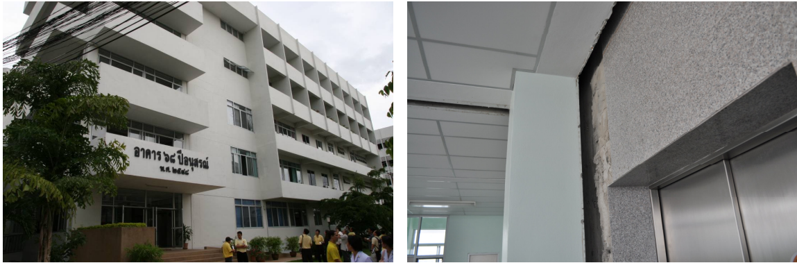
Figure 10. Damage due to pounding
