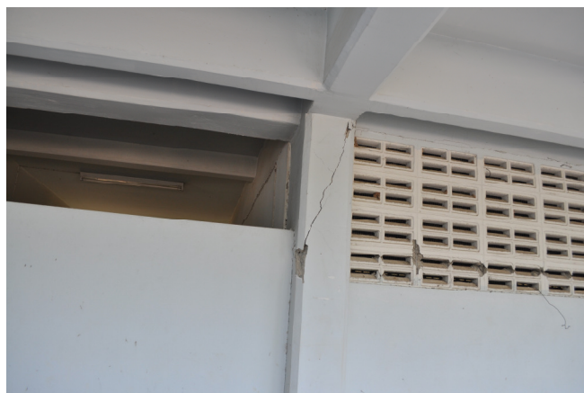
Figure 6. Shear failure of a short column
