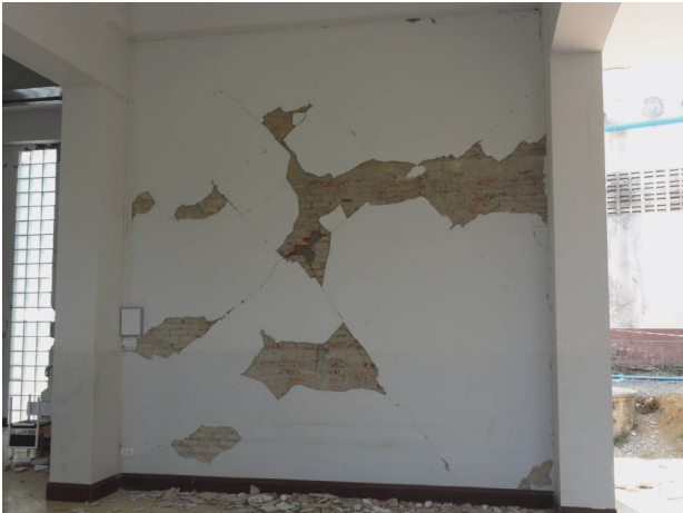
Figure 8. Diagonal cracks in a masonry wall
