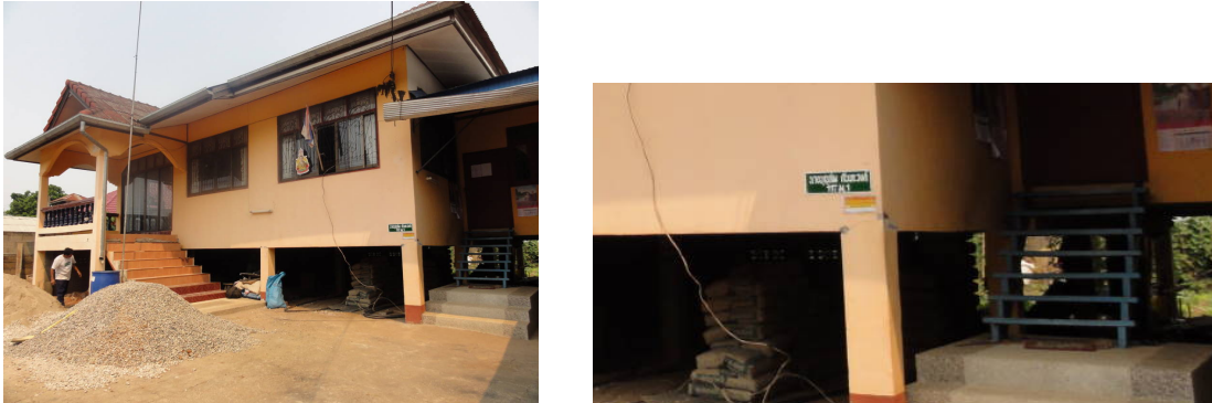
Figure 7. Damage of a building with small columns in Chiang-saen District
