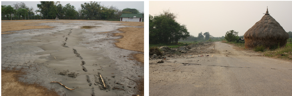
Figure 11. Liquefaction and damage to a road
