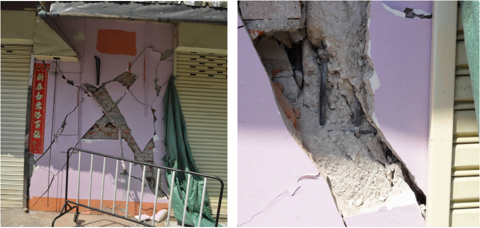
Figure 9. Damage due to load transfer from masonry walls
