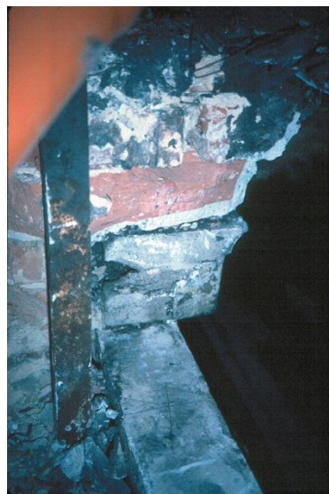
Figure 4. Partly collapsed cornice construction
