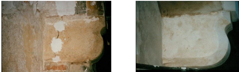
Figure 7. Assessment of a natural stone and metal cornice construction, before and after restoration
