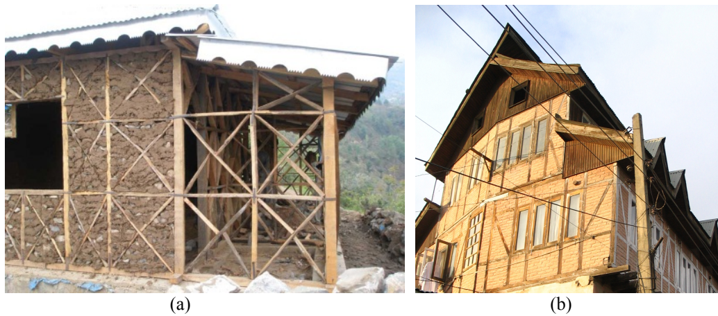
Figure 1.1 Traditional masonry for proven earthquake resistance: A system of timber laced masonry for confining masonry in small panels (Left photo source: www.e-architect.co.uk/haiti/haiti_buildings )
