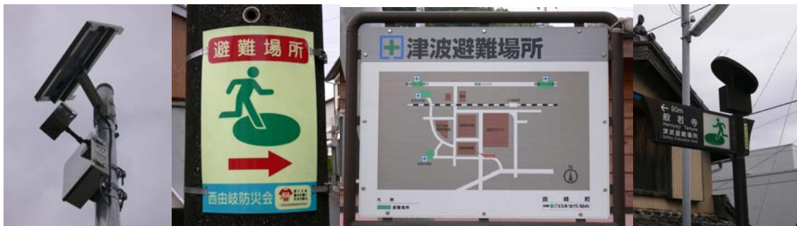
Fig.1 Outdoor disaster-prevention lighting systems.
