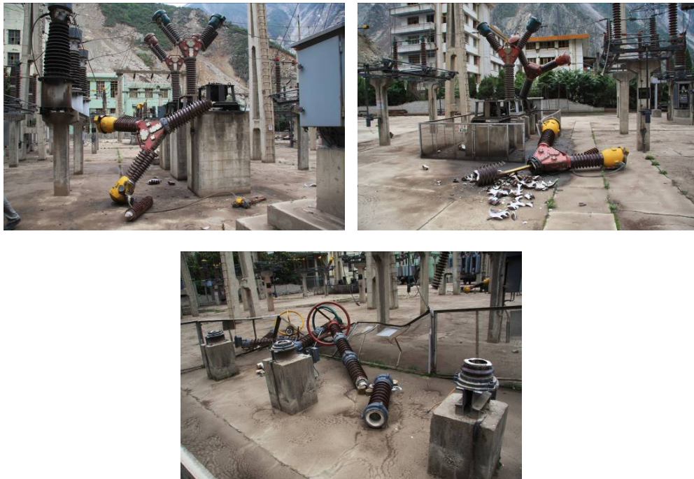
Figure 1.1 Damage to high voltage equipments in Caopo Power Plant in the 2008 Wenchuan, China earthquake [China Earthquake Administration, 2008]
