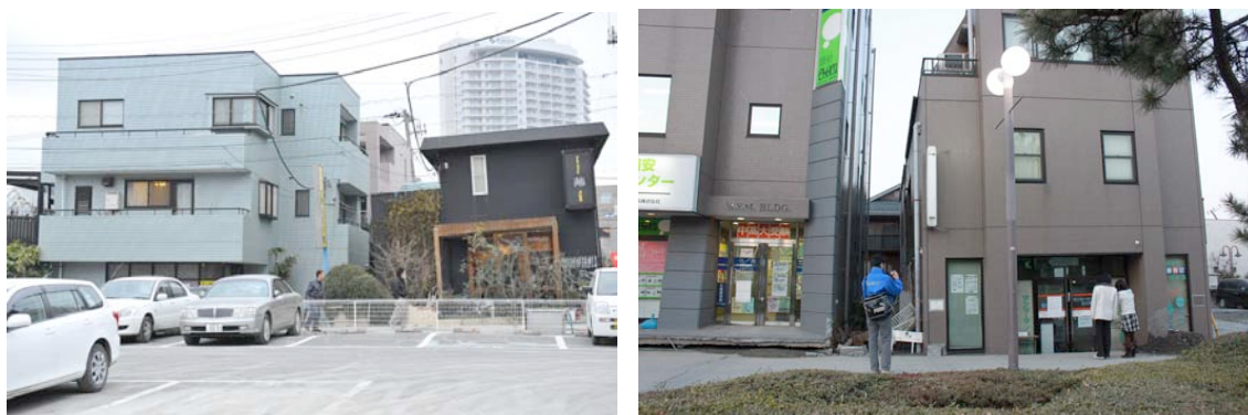
Figure 4.2. (a) Buildings suffering large settlement and tilting (left) and (b) buildings experiencing different gaps against subsiding ground (right) (Tokimatsu et al., 2011)
