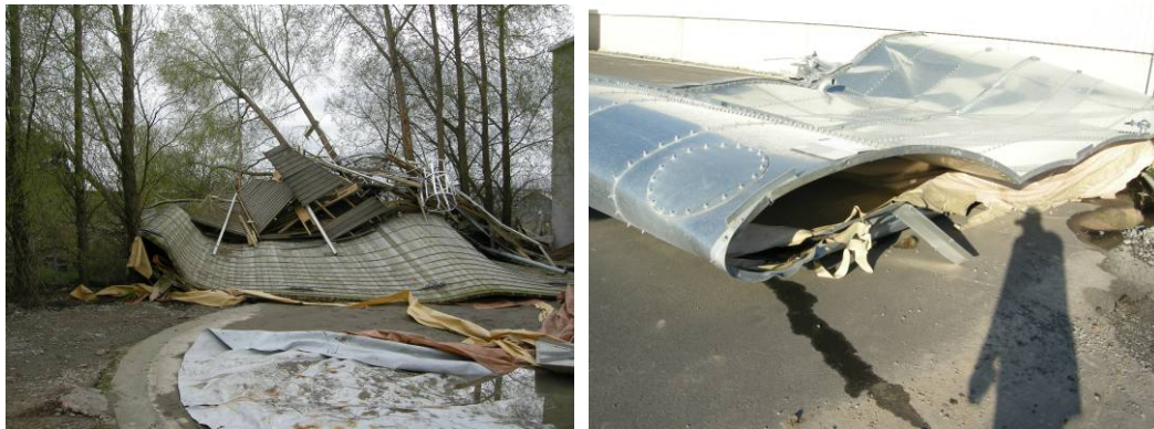
Figure 1. Total collapse of storage tanks in Darfield earthquake (2010) (Courtesy of Timbertanks).
