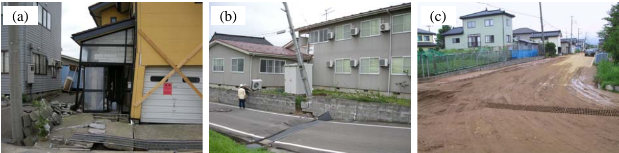
Figure 2.3. Earthquake damage in Matsunami district; (a) the severest damaged house, (b) damaged houses due to ground crack and (c) signs of liquefaction (sand boiling)
