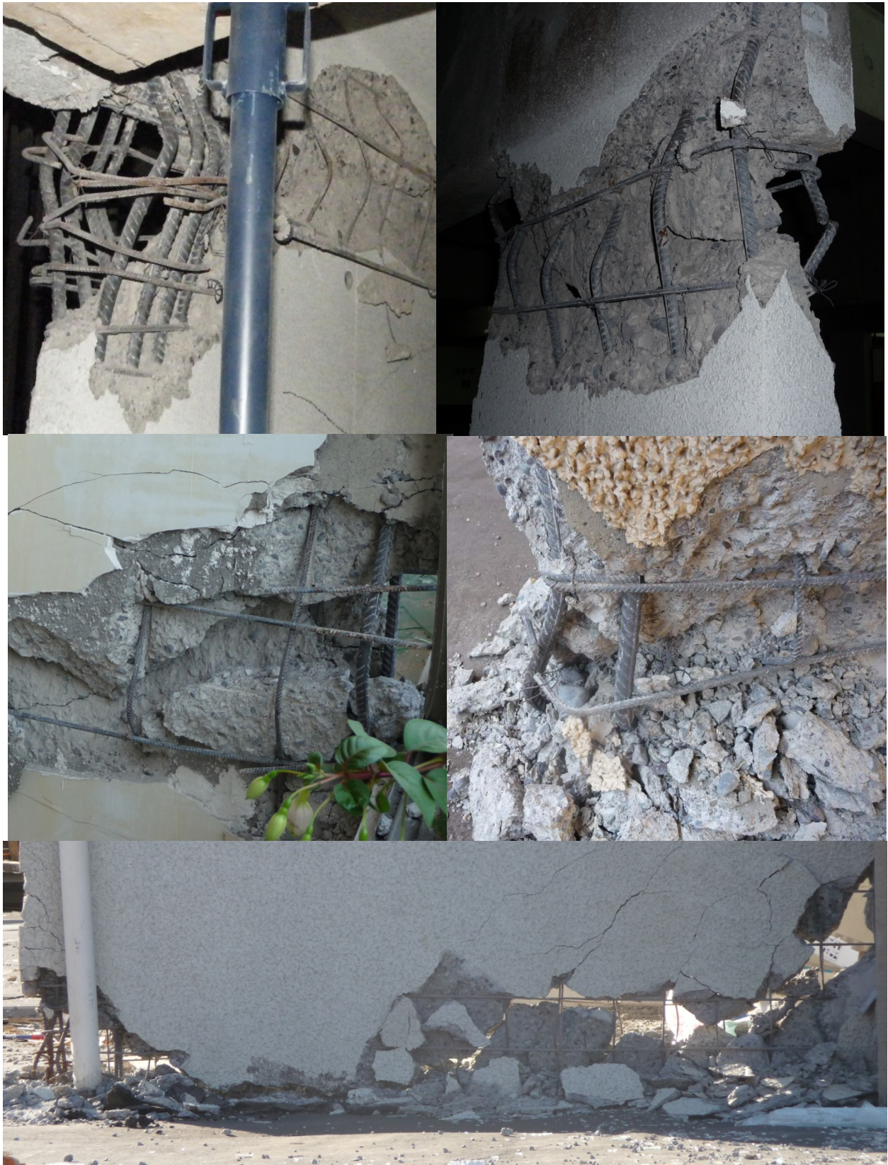
Figure 1. Compression failures of thin shear walls during the 2010 Chile Earthquake.
