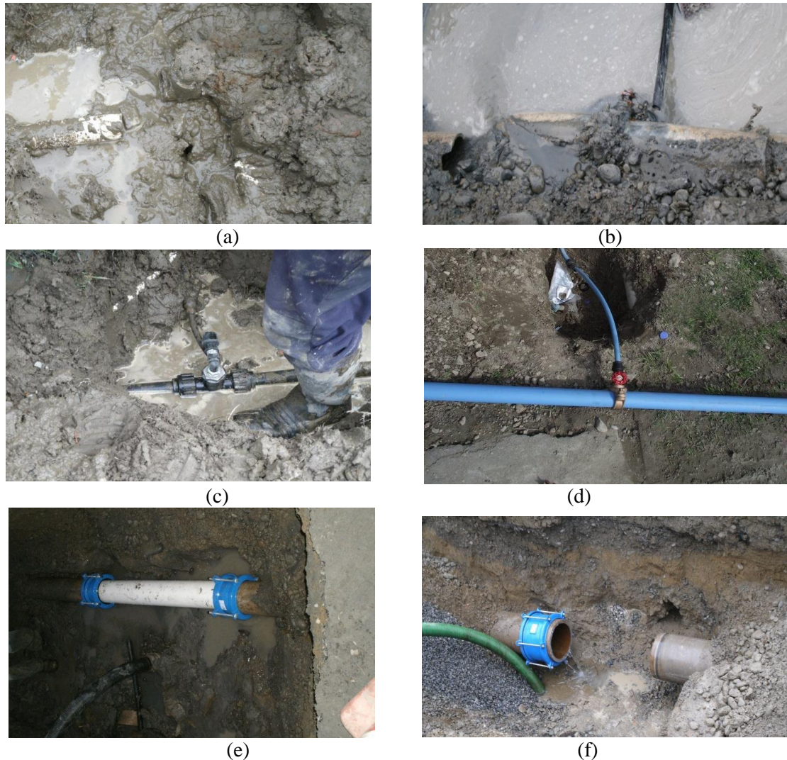
Figure 4. Pictures of damage sustained in Kaiapoi; (a) PVC main pulled away from joint due to severe lateral spreading; (b) AC main broken with broken house lateral connection; (c) disconnected house lateral; (d) temporary PE rider main installed above ground; (e) AC pipe repaired with a section of PVC; (f) water flowing out of cut open section of AC main being repaired (pictures courtesy of Ric Barber, WDC).
