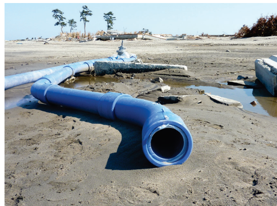
Figure 4. Damage to pipe by scouring of tsunami (Miyagi Pref.).
