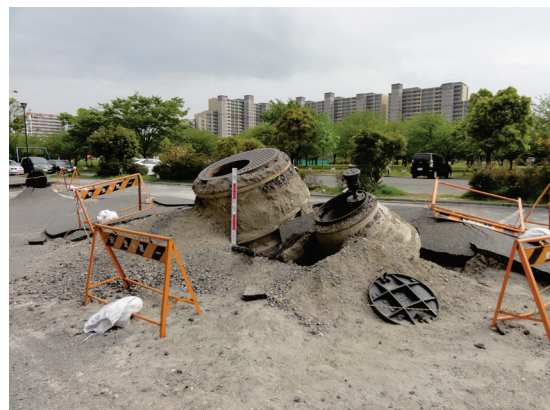
Figure 2. Uplift of underground water tank (Chiba Pref.).
