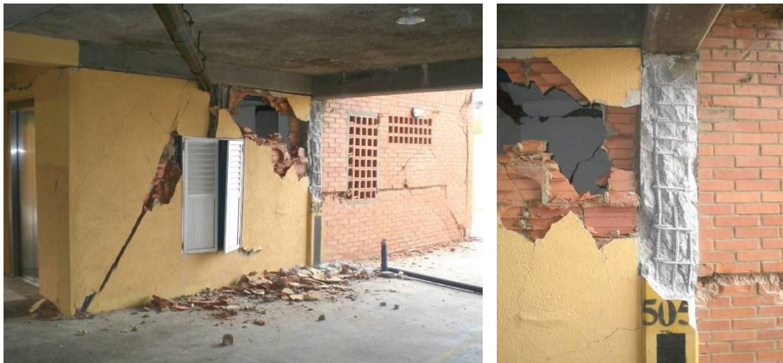
Figure 9: Short column mechanism induced after partially fails of partitions
