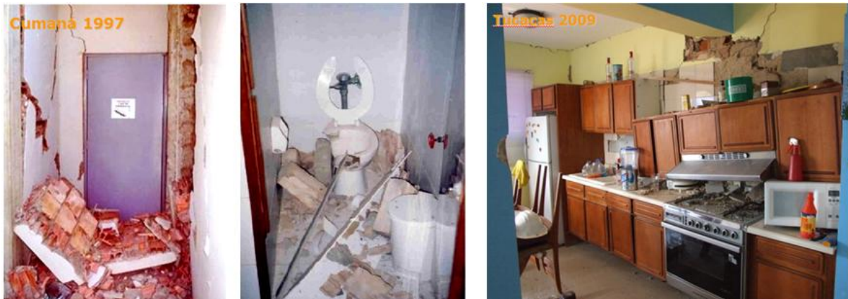
Figure 12: Risk of injury from fall of infill walls
