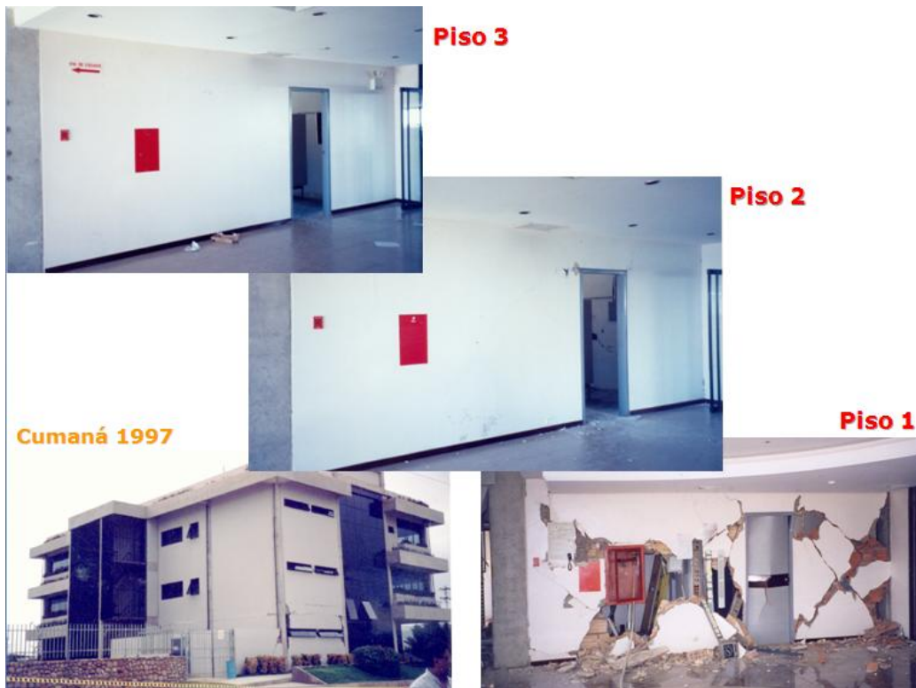
Figure 10: Soft story mechanism induced after partitions fail
