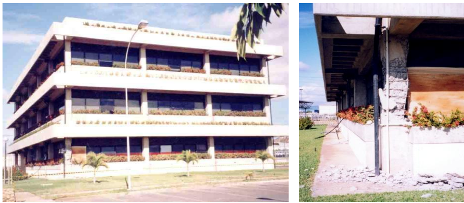
Figure 6: Effect of short column generated by reinforced concrete planters
