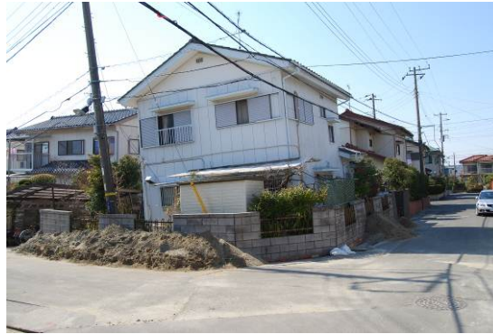
Photograph 1.1. Differential settlement of residential house in Chiba city
