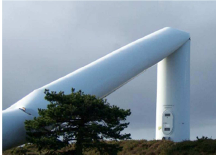
Figure 2. Example of collapse of wind turbine under wind loading. (Source: http://www.greenward-technologies.com/iso-e.htm )
