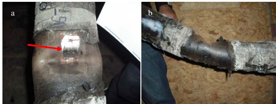
Figure 7. Wrinkling of the steel pipe section in the fix box: (a) plan view, (b) side view
