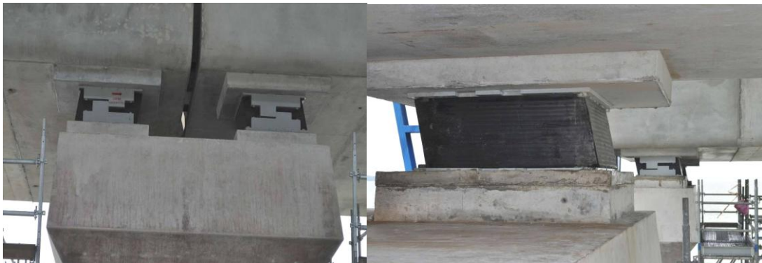
Figure 5. Left: the two end bearings (E3) of the adjacent modules installed on the pier with the locking plates in position. Right: bearing in the foreground has had the locking plates removed after being connected to structure.
