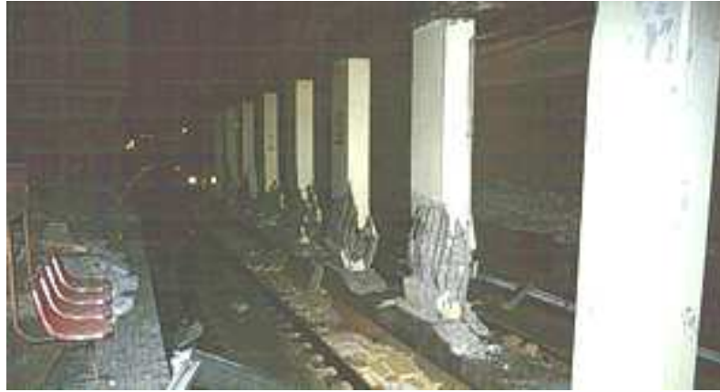
Figure 1 - Collapse of the central columns of Dakai tube station, Kobe, Japan [Iwatate, 1998]
