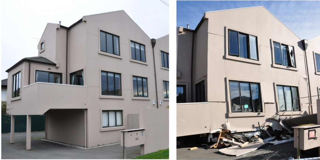
Figure 9. a) Modern wood frame home in Christchurch that experienced subtle dimpling in its finish at attachments and along edges around wall panel perimeters after the September 2010 earthquake. b) Severe damage from the February 2011 earthquake
