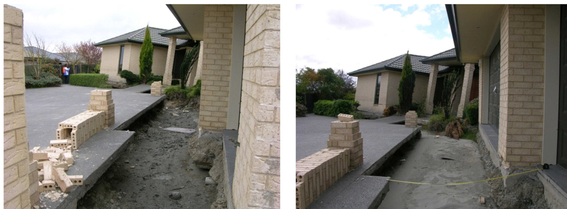
Figure 2. Damage due to sliding in Courtenay Dr.
