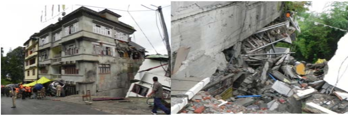
Figure 4.1 Failure at sixth storey level of a ten storey hill building during Sikkim earthquake of September 18, 2011
