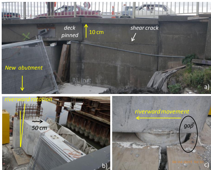
Figure 2.2. a) The front section of the east abutment has back rotated and moved upwards by 10 cm. A major horizontal crack was formed at the height of the lower part of the deck, b) The new east abutment has inclined towards the center of the bridge, c) A gap opening at the back side of the shaft due to riverward movement of the new abutment.
