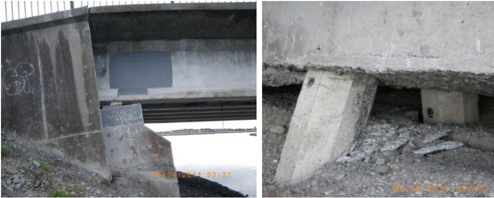
Figure 2.4. Back rotation of the west abutment of South Bridge Road Bridge around the deck and slump of the approach fill (left). Concrete spalling exposing the pile reinforcement and flexural cracks developed at the top of the piles indicating initiation of plastic hinging (right).
