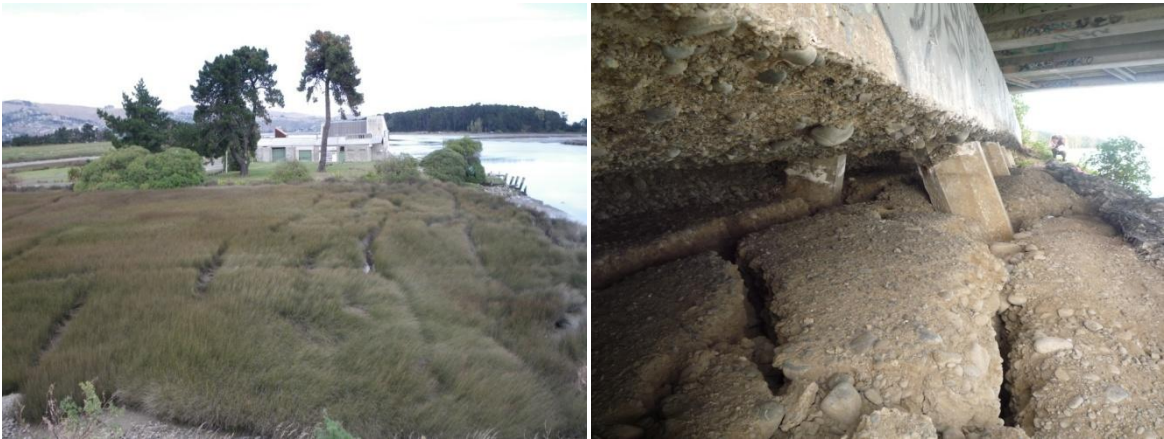
Figure 2.3. Large lateral spreading cracks in the ground parallel to the coast and adjacent to the abutments of South Bridge Road Bridge extending at a great distance inland (left). Back rotation of the west abutment around the deck and slump of the approach fill. The soil underneath the abutments has moved riverwards opening large cracks in the superficial crust and crating gaps in the front side of the piles (right).
