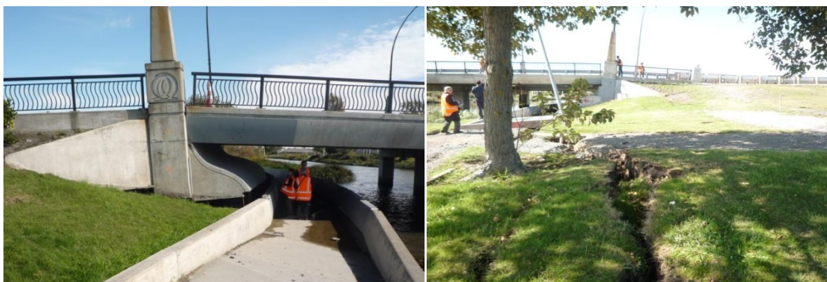
Figure 2.6. Back rotation of the abutments of Anzac Bridge and slump of the backfill. Large lateral spreading cracks in the ground parallel to Avon river coast extending in a great distance from the abutments indicating horizontal ground displacement in the free field more than 1 m.
