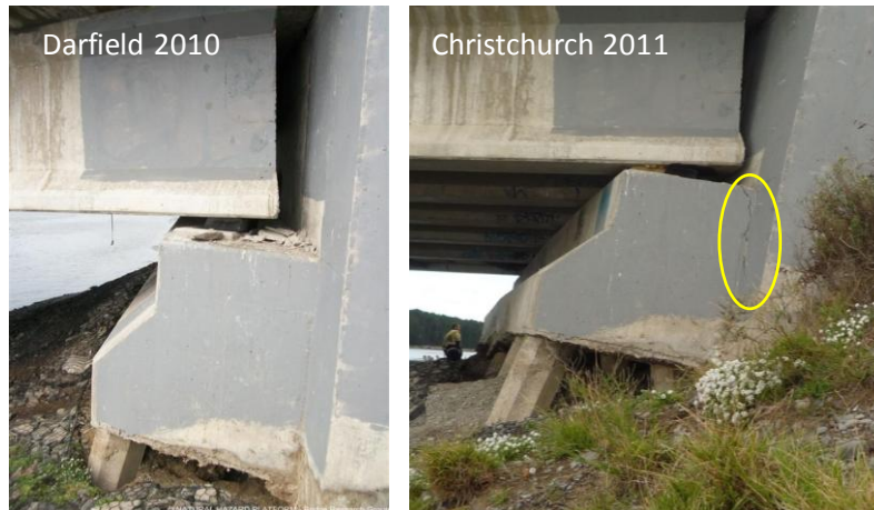
Figure 2.5. West abutment of South Bridge Road Bridge after Darfield (left) and Christchurch (right) shaking events. During Christchurch earthquake, the bridge sustained additional settlement and lateral displacements indicated by the greater exposure of the top of the pile foundation and the abutment cracks (yellow circle) in comparison to its state after Darfield earthquake (Source of left photo: NHP- Bridge Research Group).
