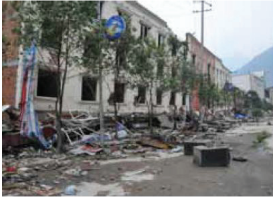
a) The collapsed first story which used as shops is very popular in Wenchuan earthquake
