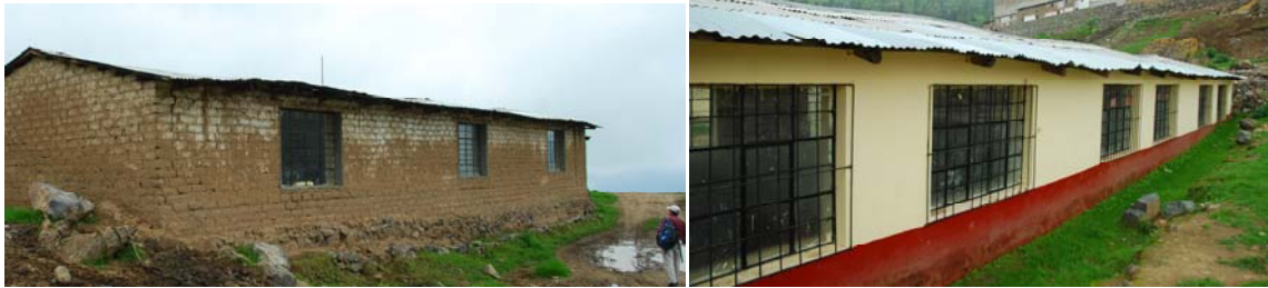
Figure 4.1. Primary school (prior to retrofit) in Chocos. The photos are of two adjacent school buildings constructed in 1954. The building on the right was selected for the retrofit project.
