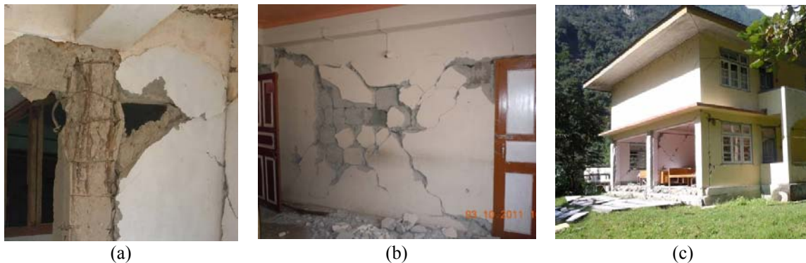
Figure 5.2 (a) Typical column failure (b) In-plane failure of weak infill masonry and (c) Out-of-plane collapse of concrete block masonry walls.
