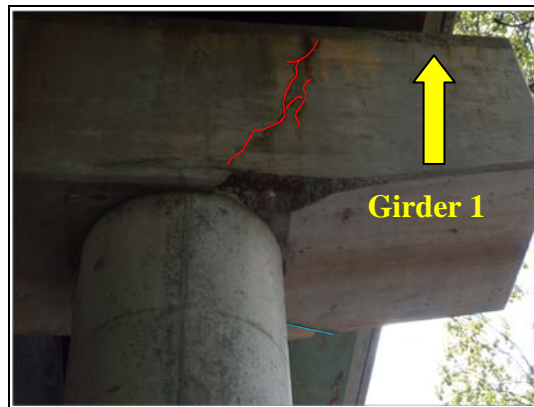
Figure 12. Pier cap crack under girder 1
