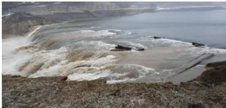
Figure 2. Dam during the earthquake
