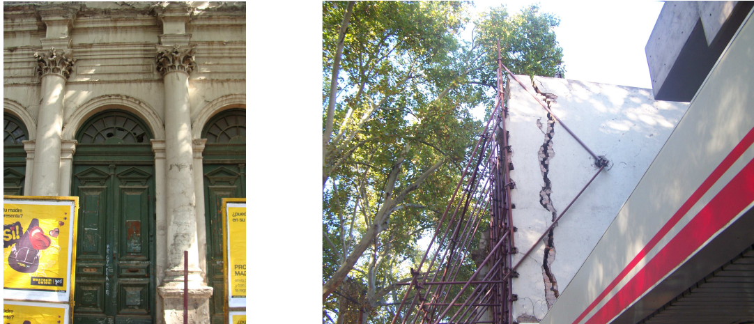
Figure 1: View of original front and the current temporary shoring.
