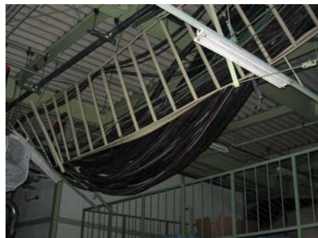
Figure 15. Failure of cable racks
