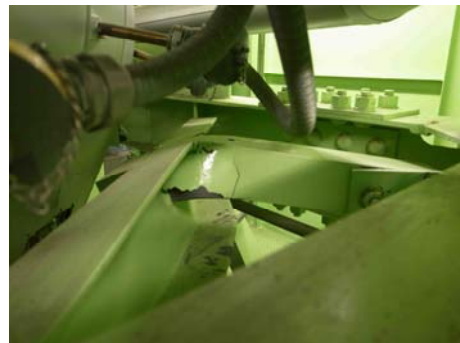
Figure 7. Damage of the anti-vibration bar of a boiler
