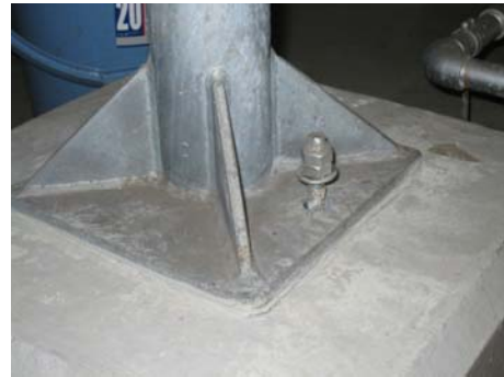
Figure 3. Deformation of an anchor bolt (Provided by JAXA)
