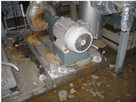
Figure 2. Damage at the base of a pump
