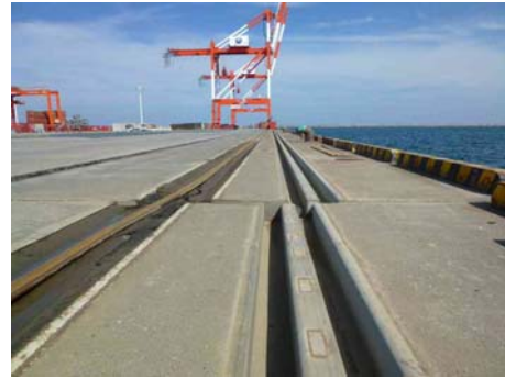
Figure 19. Quay wall deformation and misalignment of the unloader rail
