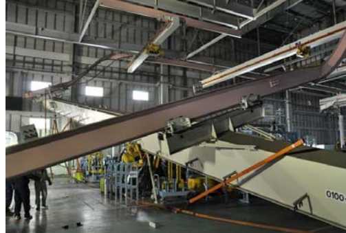
Figure 13. Failure mode of overhead crane (Fallen crane rail)
