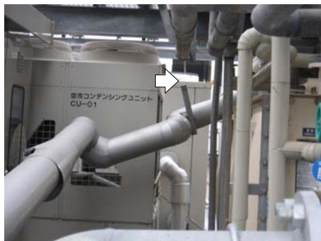
(a) In-house hanging pipe
