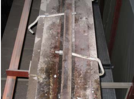
Figure 12. Failure mode of overhead crane (Damage of hook bolts, provided by JAXA)
