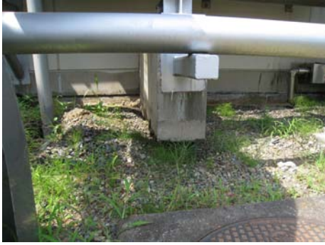
Figure 16. Pipe support hanging from a pipe due to subsidence of the soil
