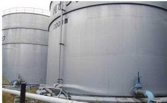
Figure 11. Buckling failure of 2,000 m 3 water tank (Thermal and Nuclear Power Engineering Society, 2011)
