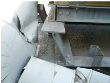
Figure 4. Deformation of the steel base of FRP tank
