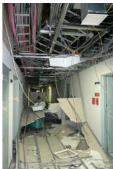
Figure 14. Failure of ceilings (Provided by JAXA)
