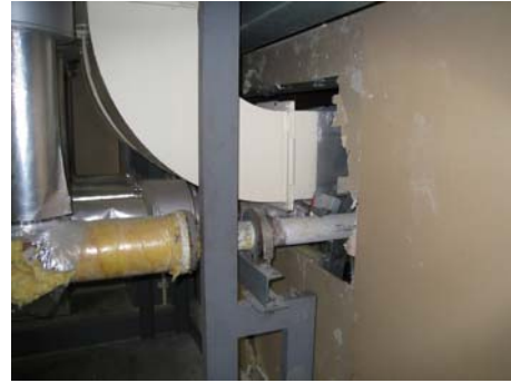
Figure 10. Damage of inner walls by pipes (Provided by JAXA)
