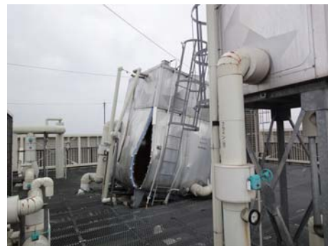
Figure 5. Failure of a water tank installed on the roof
