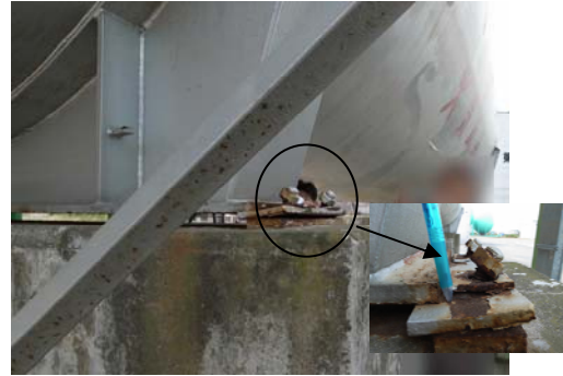
Figure 21. Lifting damage of LPG tank by tsunami
