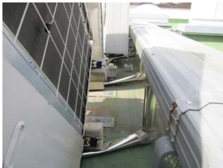
Figure 6. Tumbled equipment set on the roof
