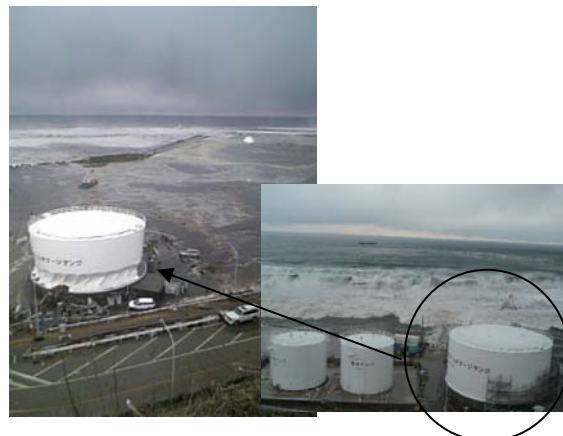
Figure 23. Buckling failure of a water tank due to the pressure of the water (Provided by TEPCO)
