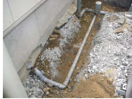
Figure 17. Buried utility pipes broken due to soil deformation
