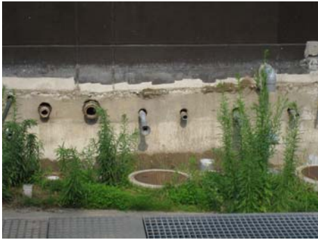
Figure 18. Pipes fractured at the connection point of the building and soil
