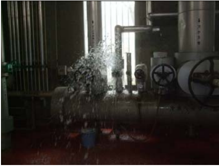
Figure 9. Failure of utility pipe and water leakage (Provided by JAXA)
