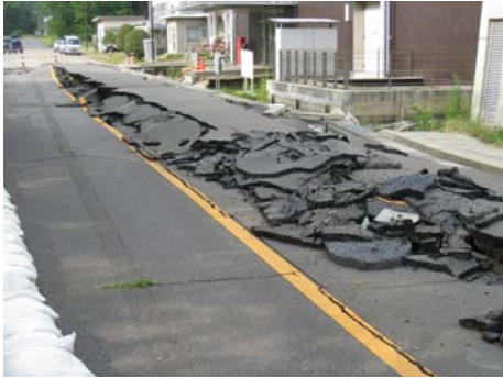
Figure 20. Damage of a road in a research facility
