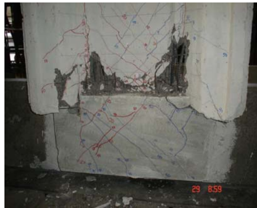
Figure 3.5. Cumulative damage of the concrete during cyclic loading tests (CLT)
