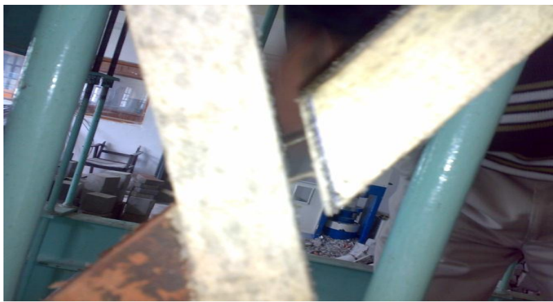
Figure 7. Brace failure in Frame 2
