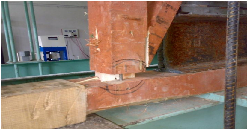
Figure 6. Joint failure in frame 2
