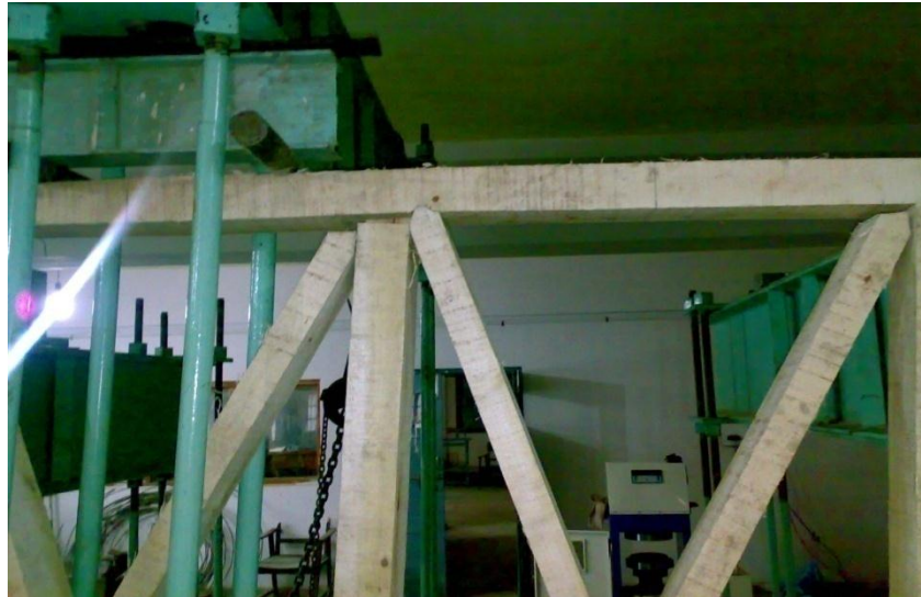
Figure 9. No joint failure in Frame 4
