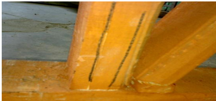
Figure 4. Vertical Cracks in the post of Frame 1
