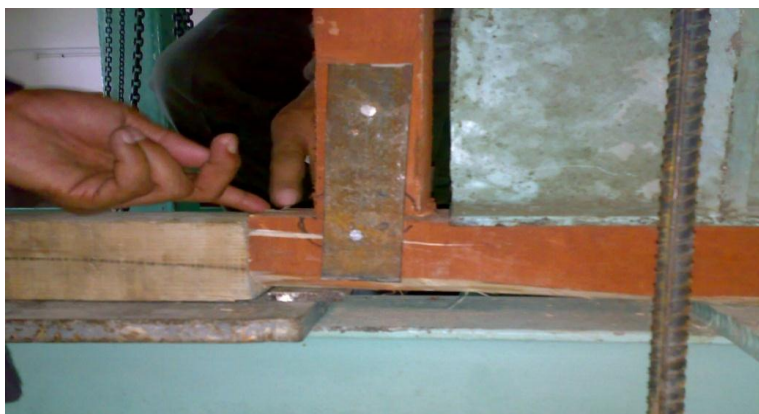
Figure 5. Bending induced in the vertical post which caused cracks at the strap levels in the line of nails
