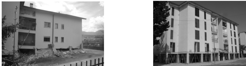
Figure 2.5. Two recent examples of severe damage attributed to the soft first story irregularity in L'Aquila earthquake, Italy in 2009, (Photos, left: Holly Razzano, Degenkolb) and in Lorca, Spain in 2011.
